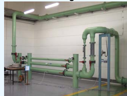
Fan Training Unit
